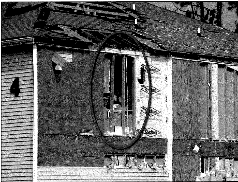
Figure 11-15. Blown-off vinyl siding and foam sheathing; some blow-off of interior gypsum board (circle). Estimated wind speed: 130 mph. Hurricane Katrina (Mississippi, 2006)
