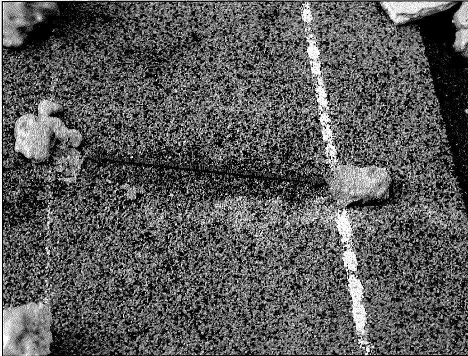
Figure 11-44. Adhesive that debonded from the cap sheet
