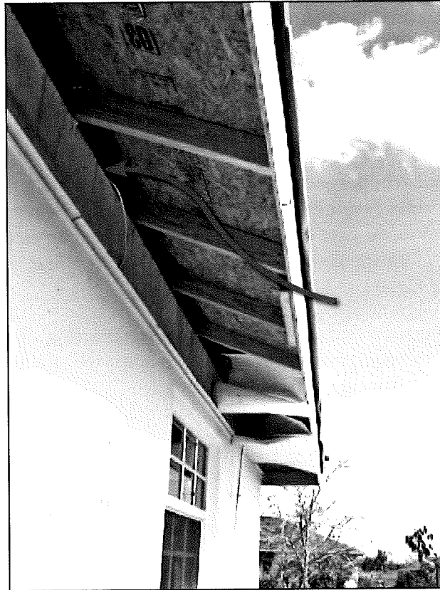
Figure 11-22. Blown-away soffit (arrow), which allowed wind-driven rain to enter the attic. Estimated wind speed: 140 to 160 mph. Hurricane Charley (Florida, 2004)
