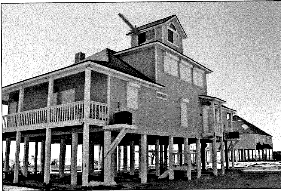
Figure 11-10. Unprotected cupola window that was broken. Estimated wind speed: 110 mph. Hurricane Ike (Texas, 2008)
