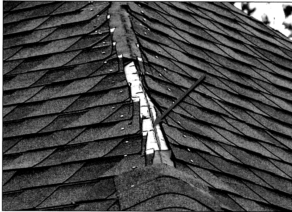
Figure 11-29. Underlayment that was not lapped over the hip; water entry possible at the sheathing joint (arrow). Estimated wind speed: 130 mph. Hurricane Katrina (Mississippi, 2005)
