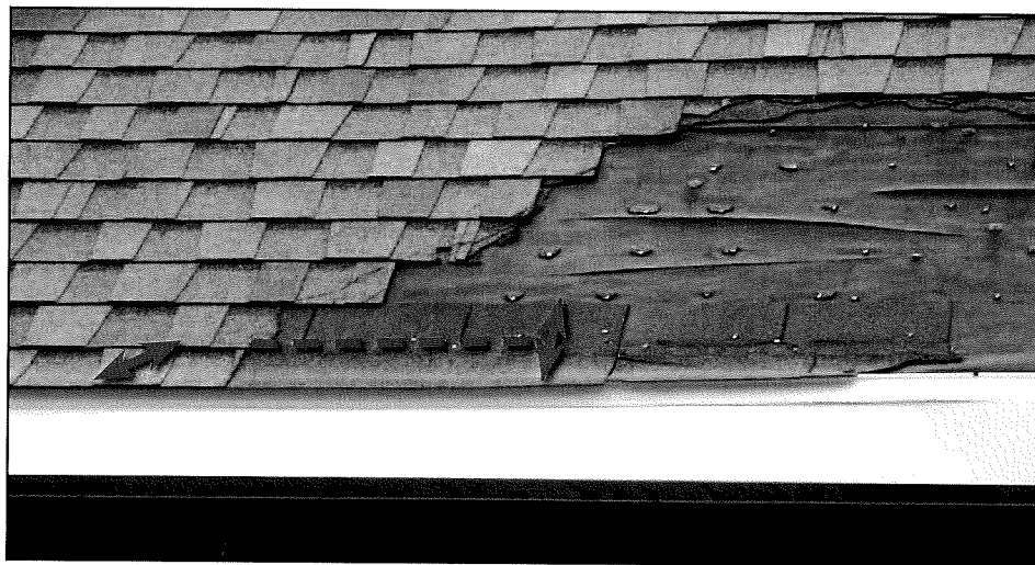
Figure 11-32. Incorrect installation of the starter course (incorrectly rotated starter, right arrow, resulted in self-seal adhesive not near the eave, dashed line). Estimated wind speed: 130 mph. Hurricane Katrina (Mississippi, 2005)
