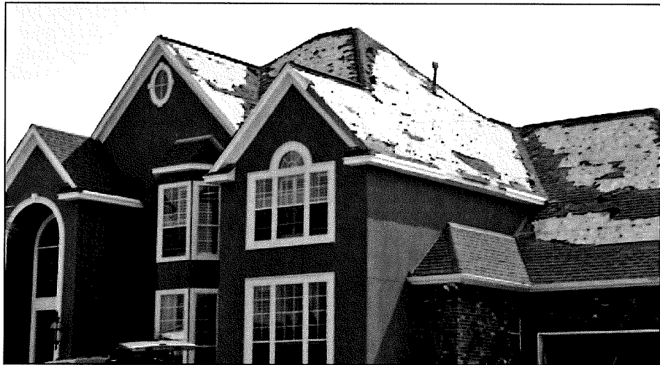
Figure 11-25. Typical underlayment attachment; underlayment blow-off is common if the shingles are blown off, as shown. Estimated wind speed: 115 mph. Hurricane Katrina (Louisiana, 2005)
