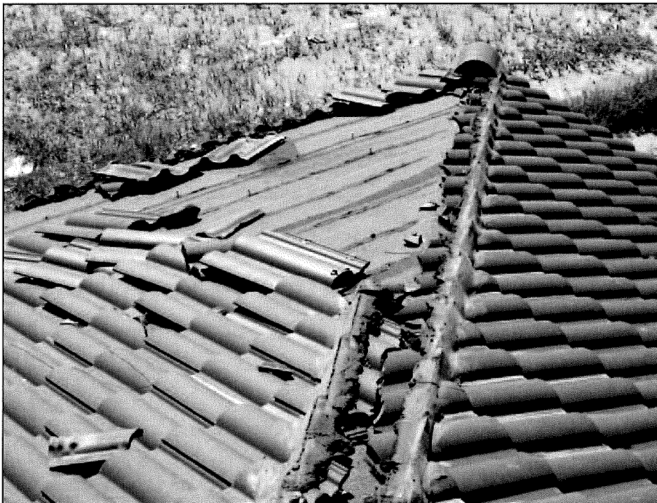
Figure 11-45. Blow-off of mechanically attached tiles. Estimated wind speed: 140 to 160 mph. Hurricane Charley (Florida, 2004)
