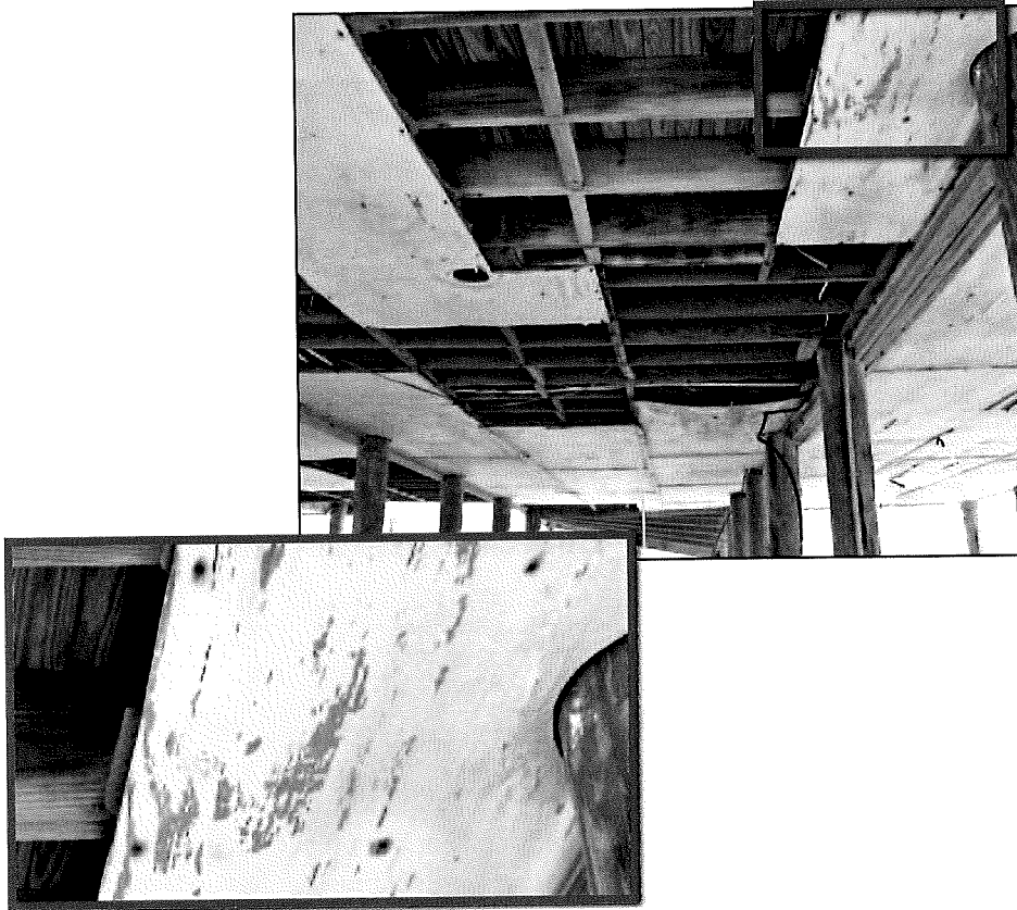
Figure 11-4. Plywood panels on the underside of a house that blew away because of excessive nail spacing. Note the corroded nails (inset). Estimated wind speed: 105 to 115 mph. Hurricane Ivan (Alabama, 2004)
