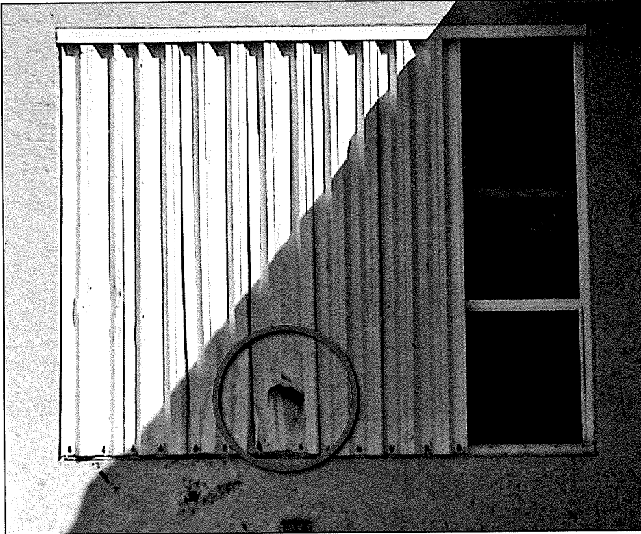
Figure 11-13. Shutter punctured by roof tile. Estimated wind speed: 140 to 160 mph. Hurricane Charley (Florida, 2004)
