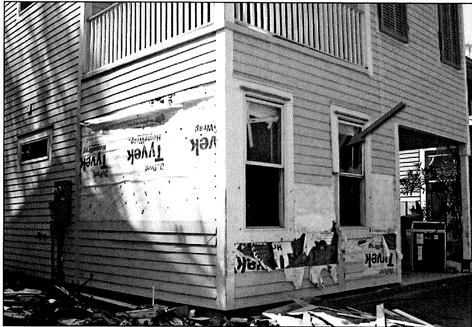
Figure 11-16. Blown-off fiber cement siding; broken window (arrow). Estimated wind speed: 125 mph. Hurricane Katrina (Mississippi, 2006)
