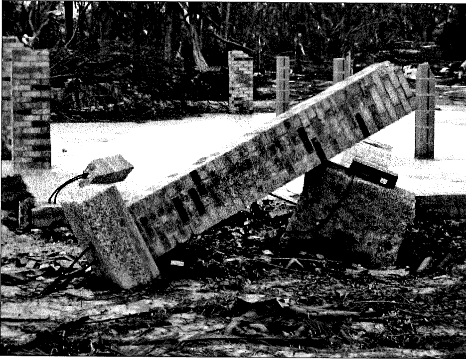
Figure 10-17. Performance comparison of pier foundations: piers on discrete footings (foreground) failed by rotating and overturning while piers on more substantial footings (in this case a concrete mat) survived Hurricane Katrina (Pass Christian, MS, 2005)
