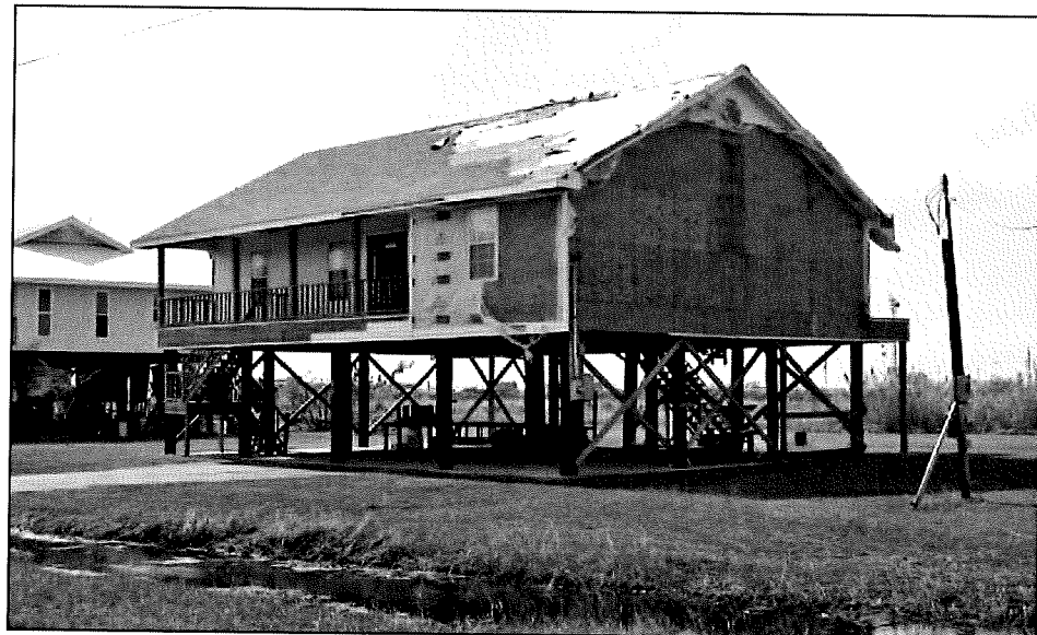
Figure 11-1. Good structural system performance but the loss of shingles, underlayment, siding, housewrap, and soffits resulted in significant interior water damage. Estimated wind speed: 125 mph. 3 Hurricane Katrina (Louisiana, 2005)
