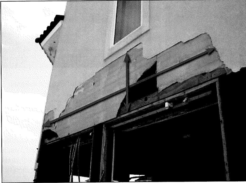
Figure 11-20. Collapse of the breakaway wall, resulting in EIFS peeling. A suitable transition detail at the top of breakaway walls avoids the type of peeling damage shown by the arrows. Estimated wind speed: 105 to 115 mph. Hurricane Ivan (Alabama, 2004)
