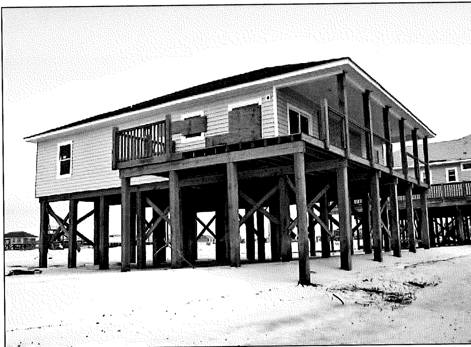
Figure 10-3. Surviving pile foundation, Hurricane Katrina (Dauphin Island, AL, 2005)
