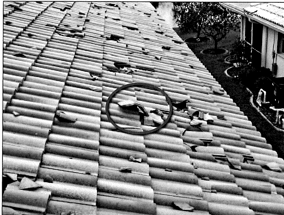
Figure 11-47. Damage to field tiles caused by tiles from another area of the roof, including a hip tile (circle). Estimated wind speed: 140 to 160 mph. Hurricane Charley (Florida, 2004)
