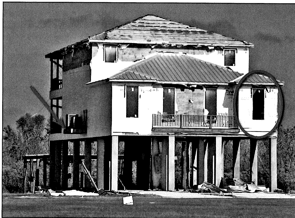
Figure 11-52. Blow-off of one of the nailers (dashed line on roof) caused panels to progressively fail; cantilevered condenser platform (arrow); broken window (circle). Estimated wind speed: 130 mph. Hurricane Katrina (Louisiana, 2005)
